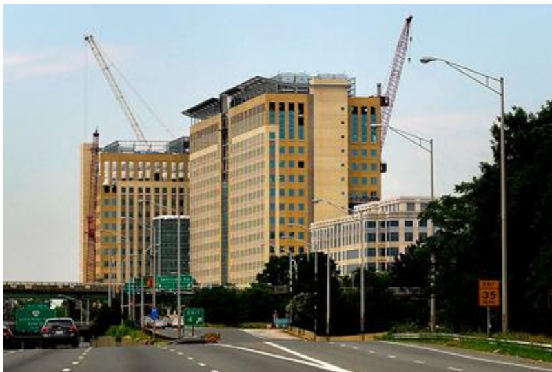
A new Defense Department office complex goes up in Alexandria. (Photo by: Michael S. Williamson / The Washington Post)
